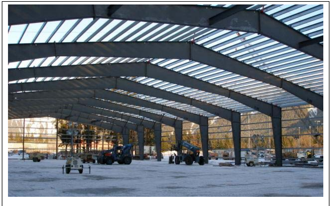
Winter construction photo of Dimond Park Field House, scheduled for completion mid-summer 2008.
